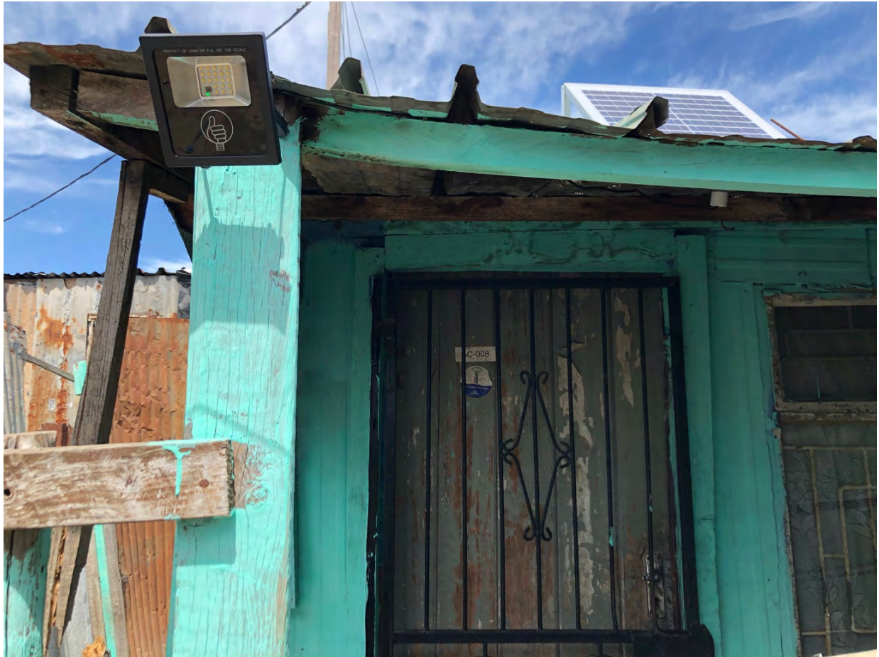
Figure 3. The solar public light installed on a household living on a treatment path
