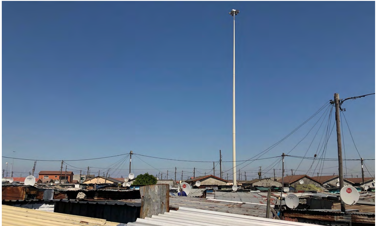
Figure 1. Picture of one of the high-mast lights serving the study site
