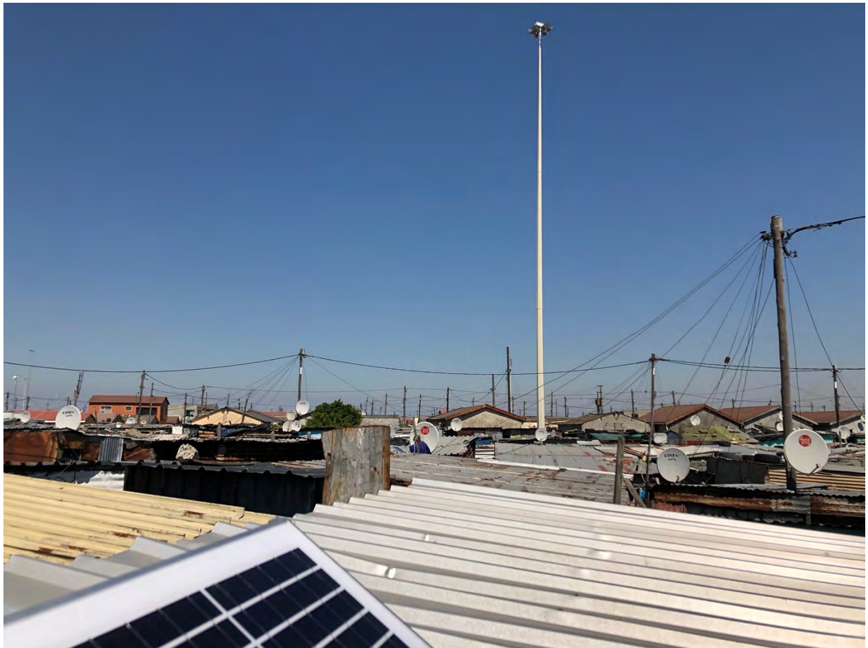
Figure 1. A high-mast light in the informal settlement
