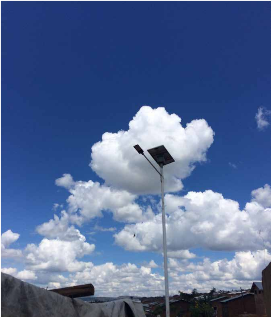
Figure 3.1. Solar streetlight in Mahama, Rwanda. © Sarah Rosenberg-Jansen.
