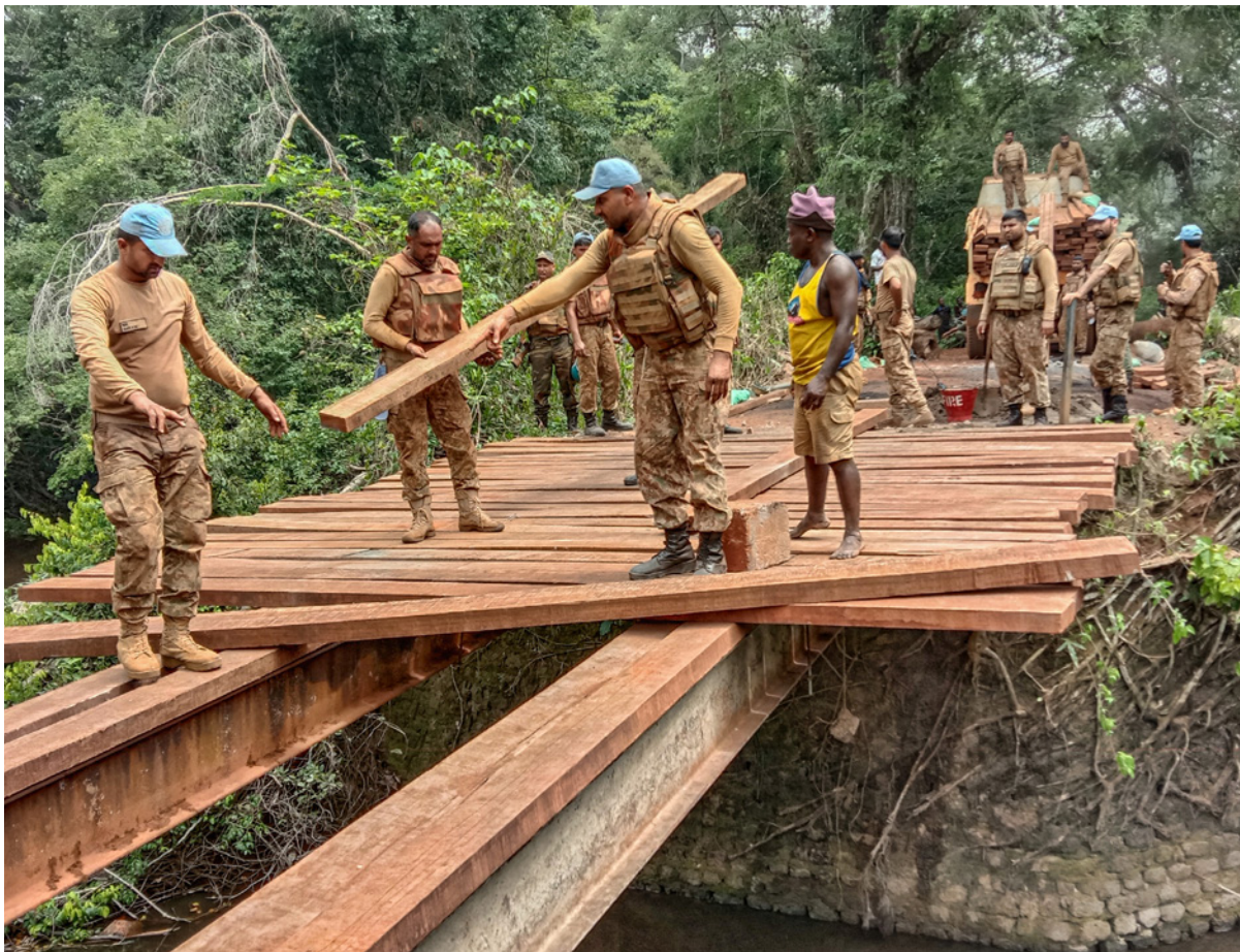
Pakistani peacekeepers work on repairing a bridge destroyed by armed groups on the Bangassou-Bakouma road. Photo by MINUSCA, 31 March 2021.
