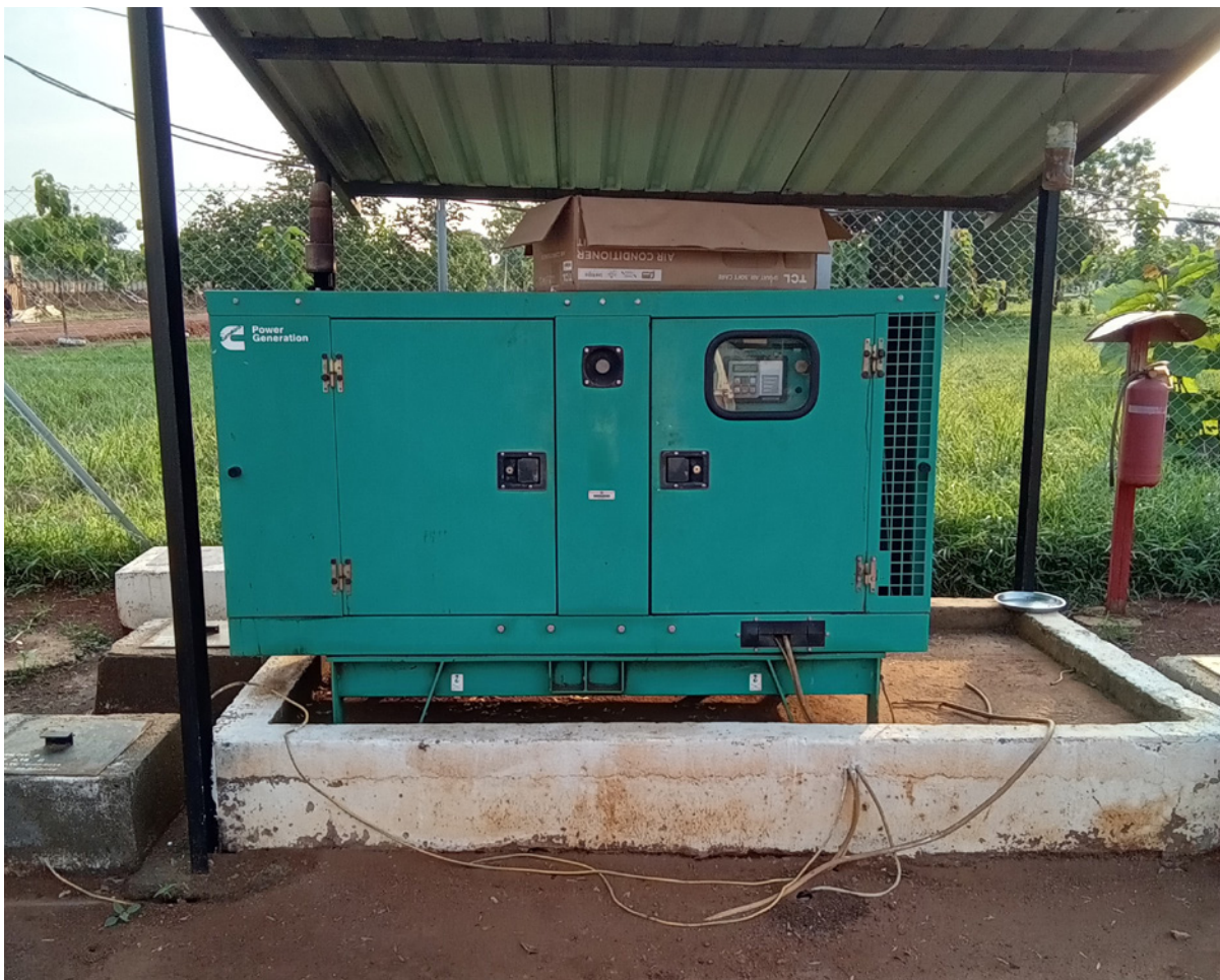
Fuel generator used by MINUSCA in Sibut (Burundian contingent). Photo by Emmanuel Singa, 7 July 2024.
